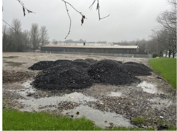
Photo 8: Rubble humps within the bare ground
